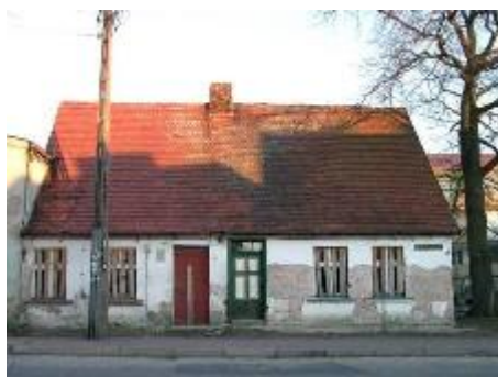
13, Kosynierów Street before rehabilitation
